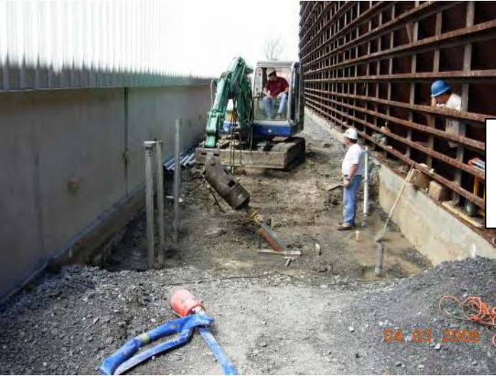
An IHI 55N mini-excavator with a 20k drive head and swivel assembly was used for the installation
